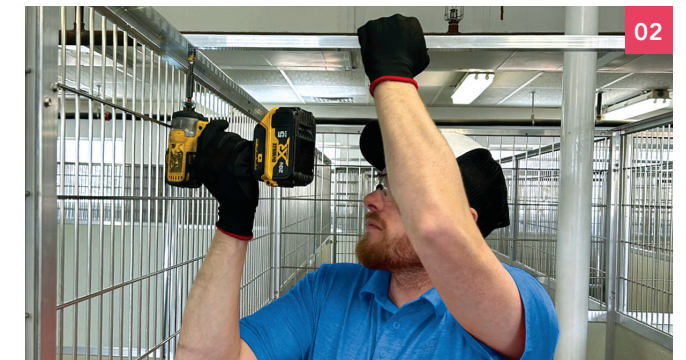
02 Appropriate hardware is installed to provide a secure fit and proper functionality.
